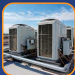
Air conditioning equipment
