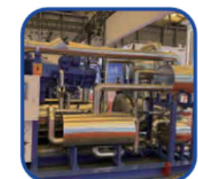
Heat pump unit
