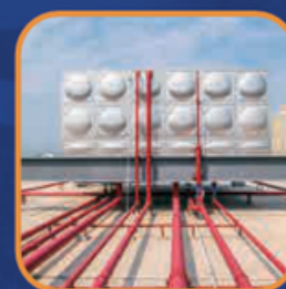
Pipe and tank measurements
